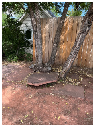
Sidewalk in critical condition on Stickney Avenue.
