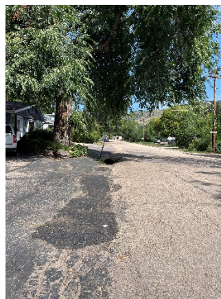
Missing sidewalk on 3 rd Avenue.
